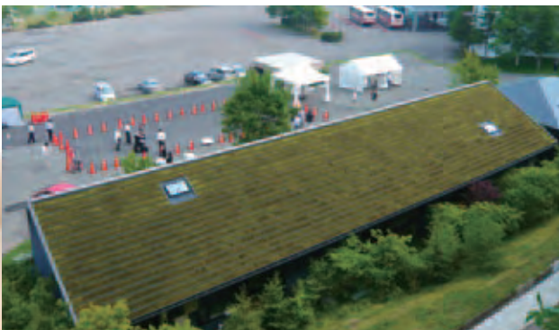
Pitched roof vegetation using Racomitrium Bridel , which limits increases in indoor temperatures and fixes CO 2
